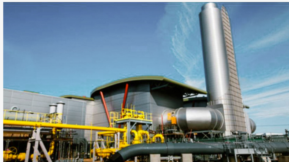
Picture 17: Langage power plant in the UK
