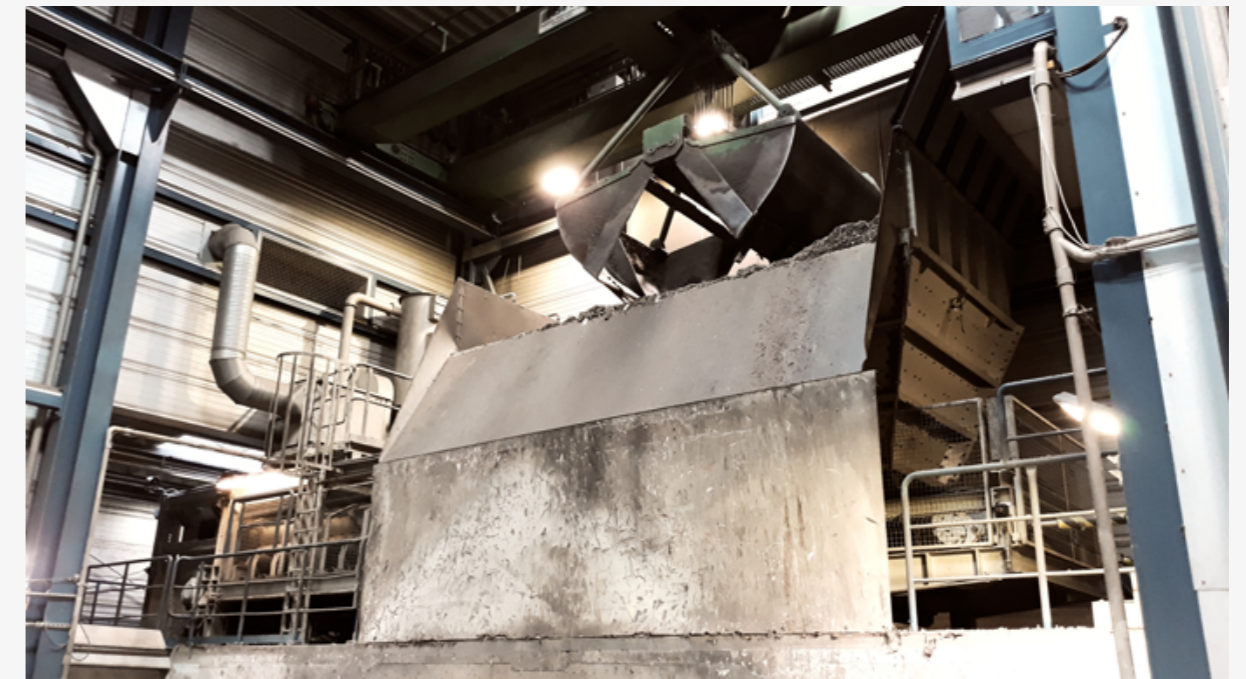
Picture 15: Waste loading and incineration from Ostrava at Schwarze Pumpe (LEAG)
