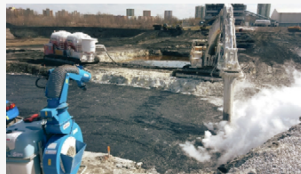
Picture 13: Treatment of the sludge
